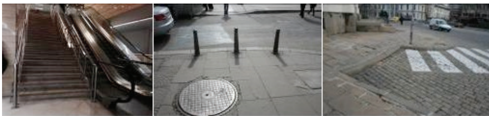
Figure 1. Images of a few examples of non-compliance with regulations. Photo 1. Lack of elevator or platform at the exit of the newly built subway station Sofia University "St. Kl. Ohridski "by the side of the King's Garden; Photo 2. Lack of tactile ground and insufficient space for crossing on Blvd. "Vitosha"; Photo 3. Crosswalk ending with high curb at one of the entrances of the church "St. Al. Nevsky"
